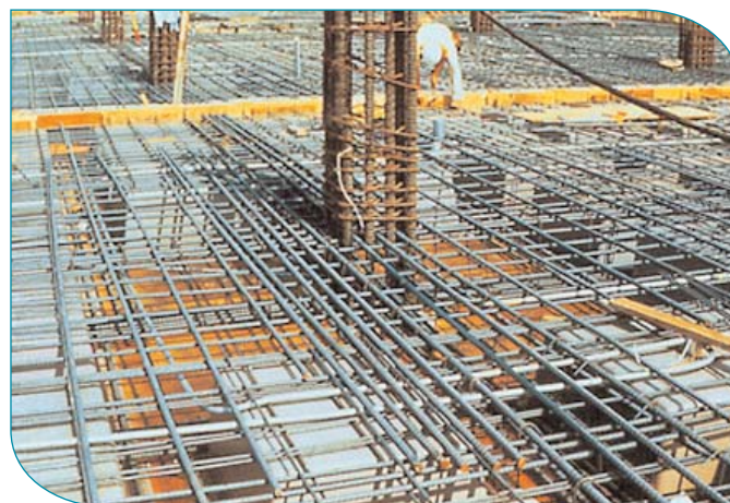
Figure 8. Continuous column strip bottom bars through the column core give the slab some residual capacity in case punching shear failure at a single support.[13.3.8.5]
