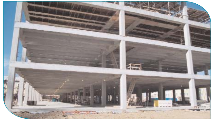
Figure 1. Perimeter beams with continuous top and bottom reinforcement provide continuous tie around the structure.
